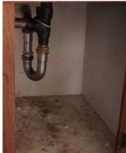
Leaks from plumbing faults
